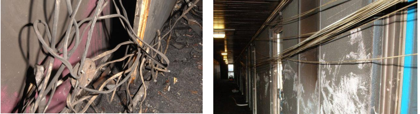
Figure 5 Fallen cable at Shirley Towers
